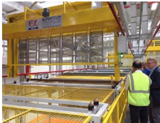
Paint facility at the new production plant in Manisa, Turkey, opened in 2018.
