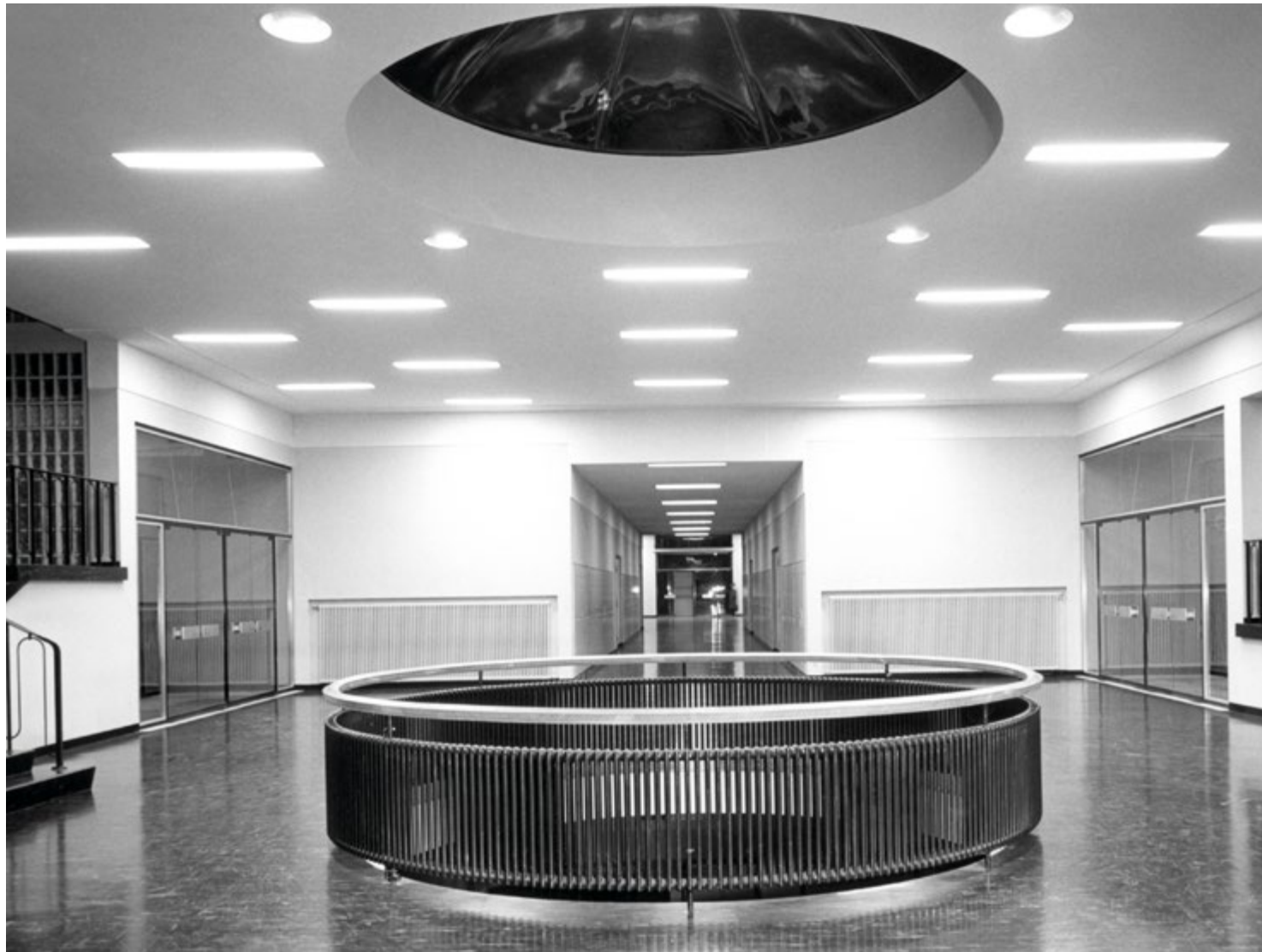
On request, the Zehnder radiator was also available bent or angled. The picture from the Lavey-les-Bains school near St-Maurice shows the radiator in an architectural function as a railing.
